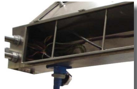
Overhead Wiring Trough
