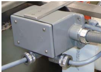
Painted Junction Boxes
