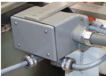
Painted Junction Boxes
