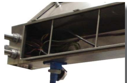
Overhead Wiring Trough
