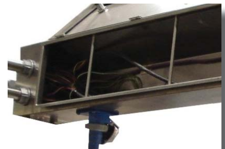
Overhead Wiring Trough
