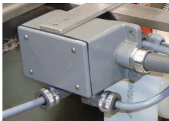
Painted Junction Boxes
